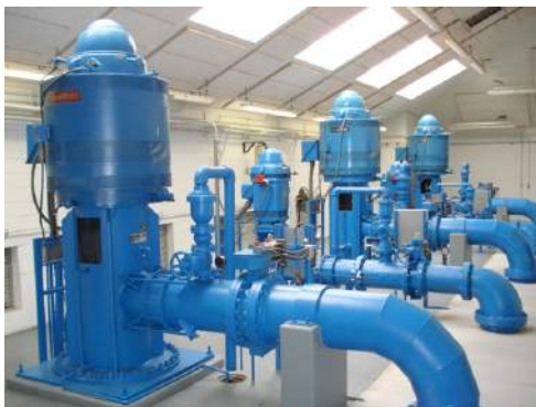
Pumps in the Celestial Road Pump Station
